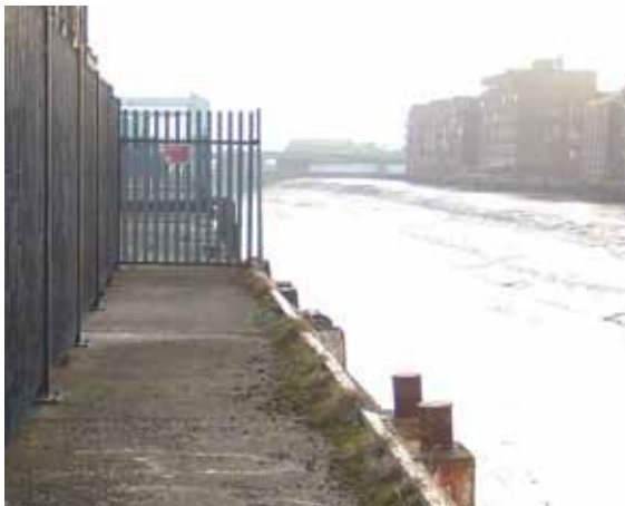
PRoW No.11 River Hull Examples of obstructions (above, above right)
