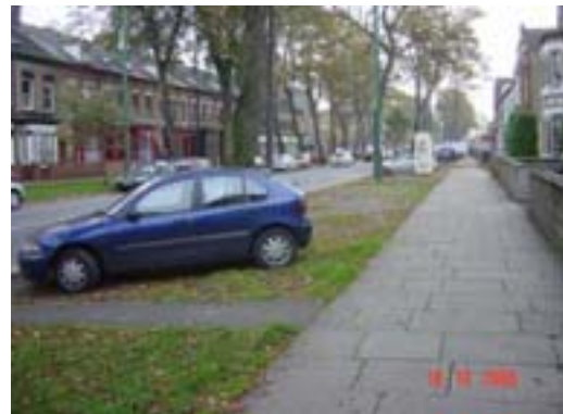
fig 24 York stone pavers, south of Newton Street, erosion of verges by parked cars.
