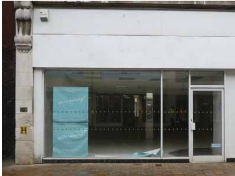
Out of proportion plate glass shop front with an overly deep fascia
