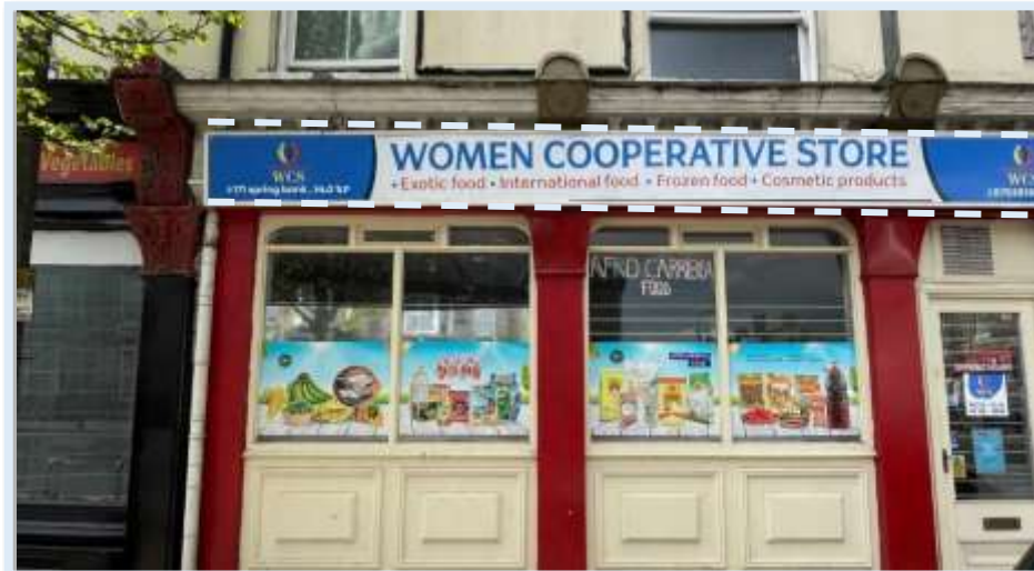
Figure 110 171 Spring Bank showing how the fascia sign is the correct depth but extends over the corbel detail (Author, 2023)
