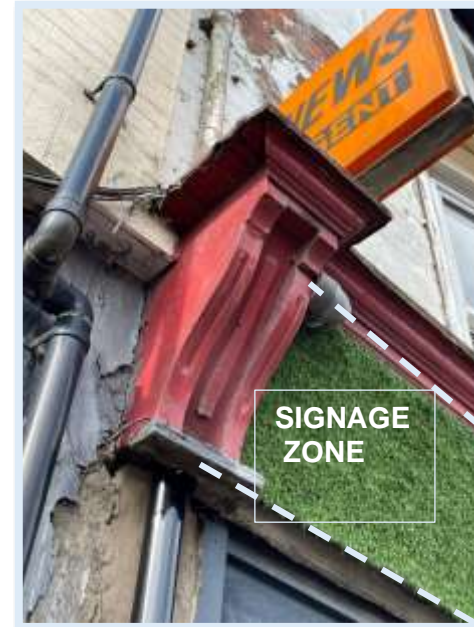
Figure 108 - 21 Spring Bank with the original corbels, cornice and fascia sign board retained (Author, 2023)
