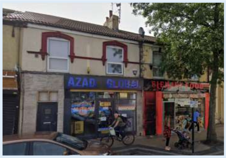
Figure 105 - All of the original shopfront has been removed and replaced with new metal framed shopfronts and low quality side doors to upper floor residential. (Google Maps, 2009)
