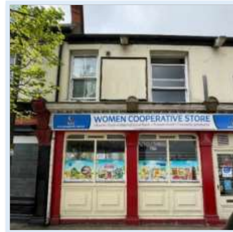
Figure 101 - 171 Spring Bank has retained its historic shopfront but has suffered from intrusive signage and loss of decorative corbels. (Author, 2023)
