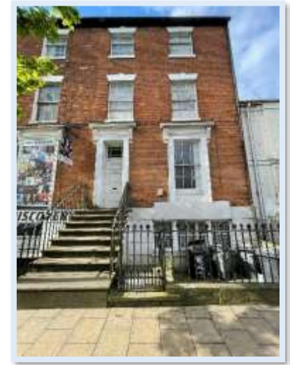
Figure 71 - The use of terracotta brickwork to the Georgian buildings at 53-55 Spring Bank built prior to 1830. (Author, 2023)
