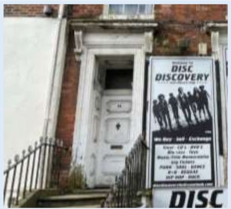
Figure 92 - Original doorway entrance and portico with scroll details and plaster surround (Author, 2023)
