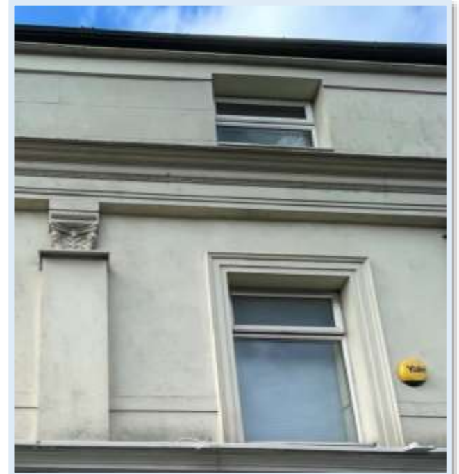
Figure 78 - Externally applied insulation and render applied externally to the external walls of Stone Boy House. (Author, 2023)
