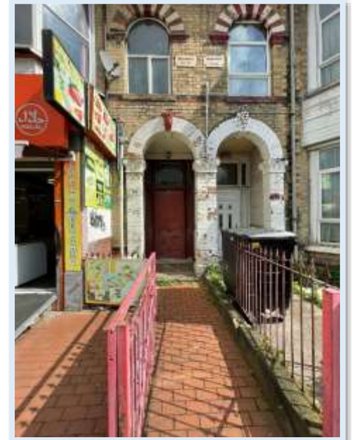
Figure 87 - Low quality modern metal railings to the LHS and original decorative railings to the RHS of the primary entrance. (Author, 2023)
