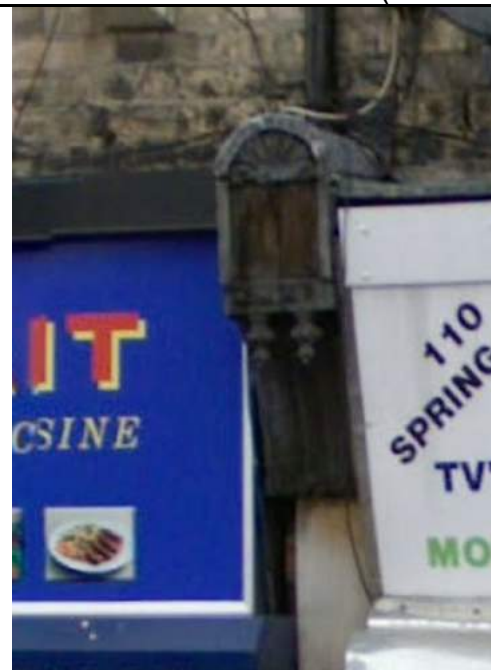
Image from 2008 showing the original timber corbel detail between No 110 and 112 (Source – www.google.co.uk/maps )
