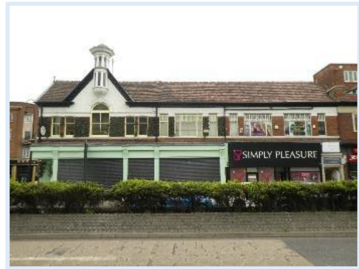
Figure 52 'In-active and poor-quality shop front to Ferensway House
