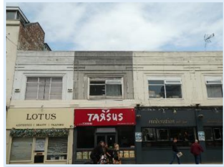
Figure 64 Loss of Uniform Appearance of Windows on South Street
