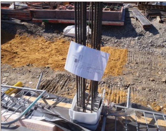
Figure A4.9 On site schematics to aid construction workers build the gas protection system (courtesy Alderburgh Group)
