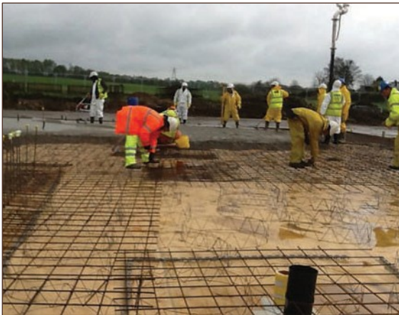
Figure A4.57 Unprotected gas membrane damaged by heavy traffic (courtesy MEC Environmental Ltd)
