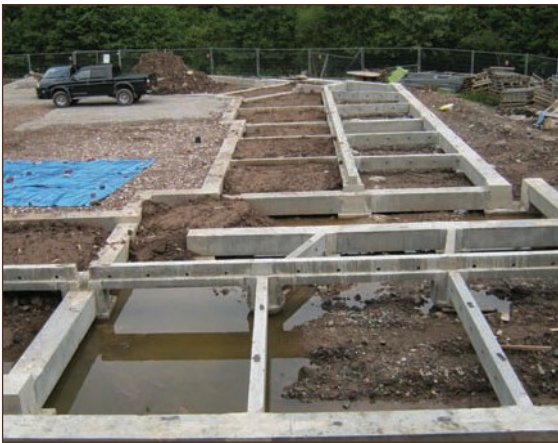
Figure A4.33 Good ventilation in internal sleeper walls, cast into prefabricated beams (courtesy Smith Grant)
