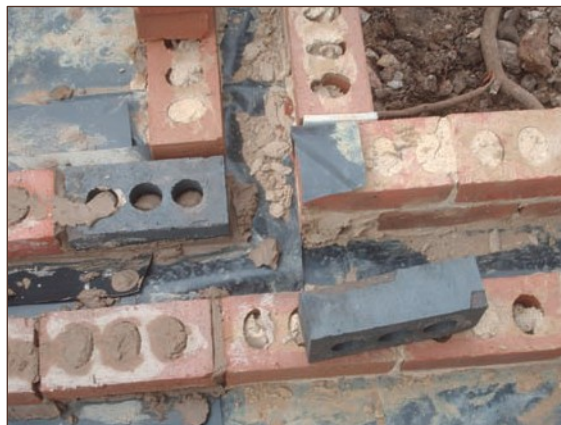
Figure A4.66 Follow-on trades proceeded work before gas membrane joints sealed (courtesy Card Geotechnics Limited)
