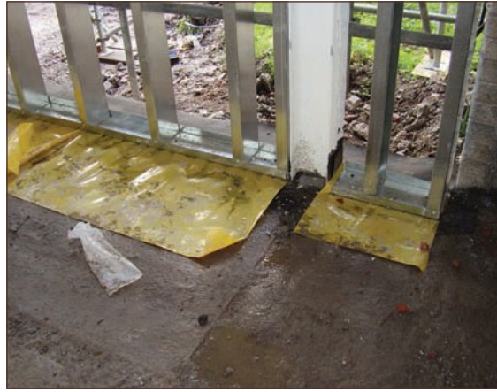
Figure A4.80 Column left unsealed (courtesy PAGEotechnical Ltd)
