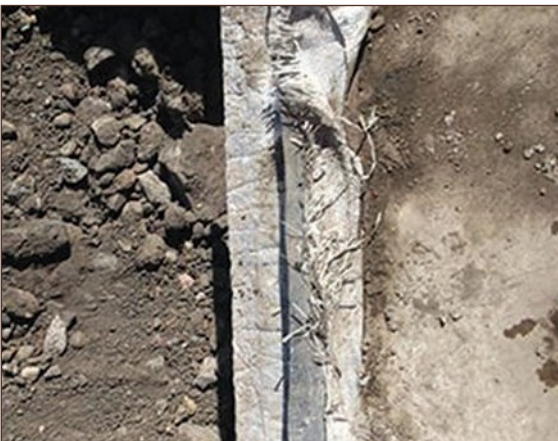
Figure A4.53 Gas membrane left exposed for long period of time, shows significant fraying at cavity edge (courtesy NHBC)
