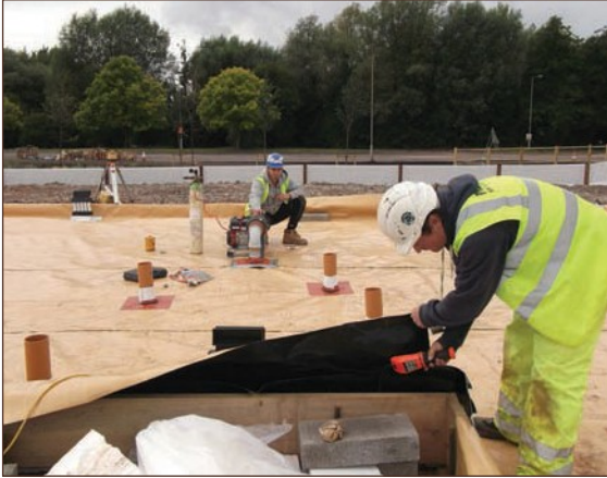
Figure A4.37 Tracer gas testing, whereby gas or smoke is applied under pressure beneath the installed gas membrane and detectors are used to screen for leaks above (courtesy NHBC)
