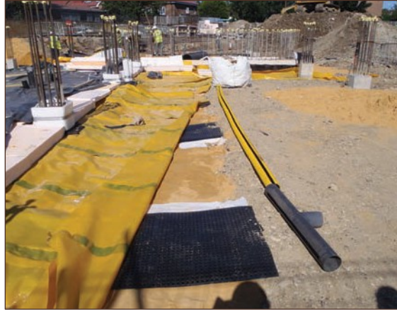
Figure A4.8 Geotext beneath the 2000g taped gas membrane lined up with collector pipes (courtesy Alderburgh Group)
