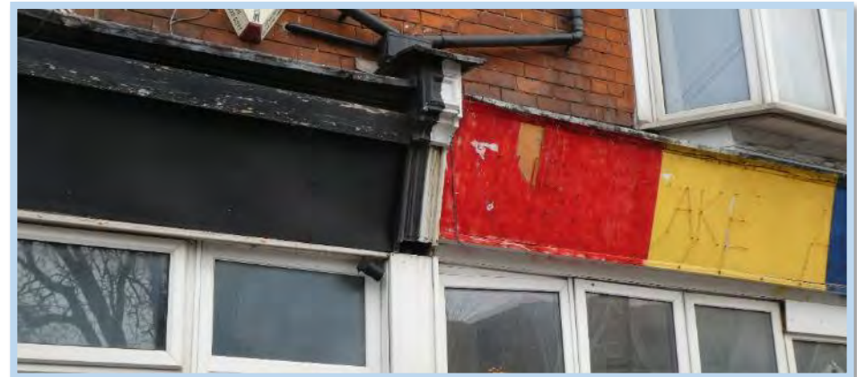
Figure 77 Remain sections of capitals and fascia at Nos. 438 and 440, but shop front replaced in 20th century.
