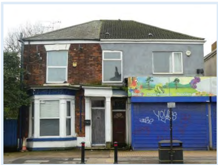
Figure 208 Potential to restore a residential façade and remove a poor-quality shop frontage at Nos.201-203
