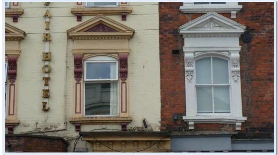
Figure 119 Richly decorated windows at Nos.327-43, but loss of uniform window joinery.
