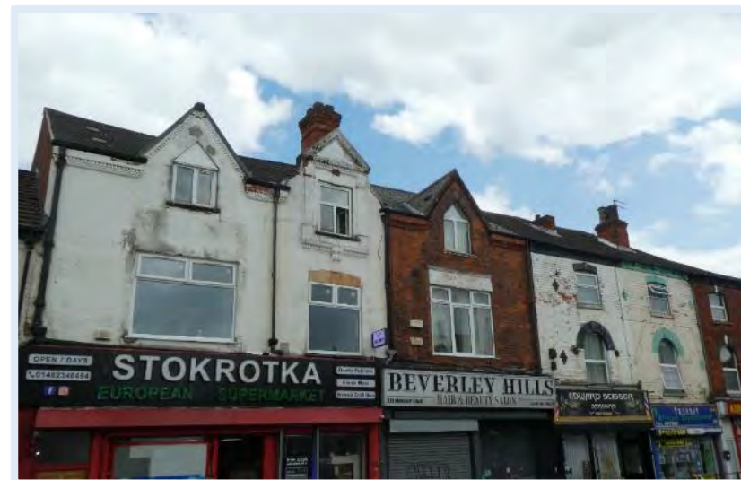
Figure 123 Poor quality windows in the Stepney area.
