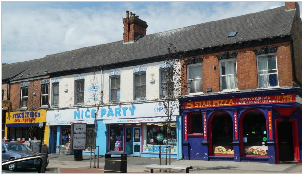
Figure 22. Examples of negative elements in shopfronts such as oversized facias and cluttered advertisements.
